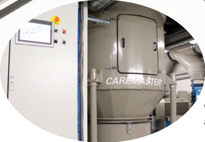
Vacuum blower and filter system
