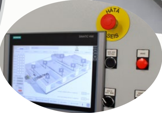
Control system / remote SCADA connection
