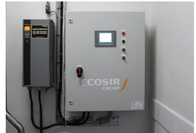
Vacuum system control unit with frequency inverter (VLT)
