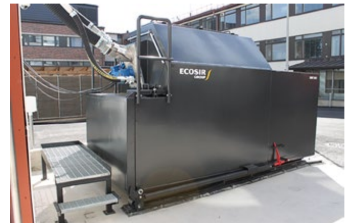
Waste vacuum container (outdoor)
